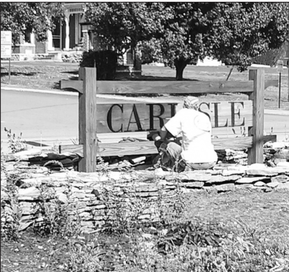
Photo by Jeremian Brown Dorsey Watkins was out at the Triangle Park putting another coat of sealant on the dign and digging a ditch for the electric to install a spot light.
