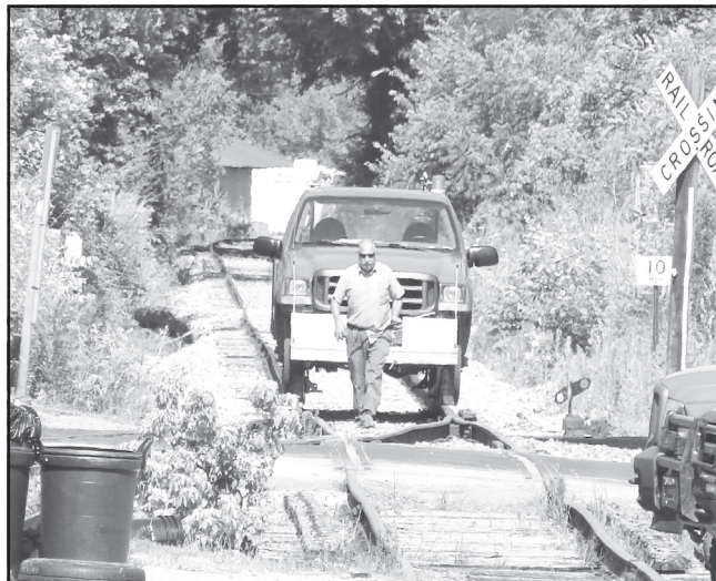
Left: A TTI railroad worker checks the width of the track near the intersection with Upper Jackstown Road. Today the railroad is owned by CSX and has its terminal in Maysville. The railroad is used largely for the transportation of coal from the mountains of Eastern Kentucky to Maysville and barges on the Ohio River.
