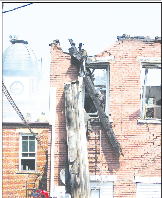
Photo by Cecil Lawson This is some of the extensive damage done to 224/226 N. Locust St. in last Fridays fire.
