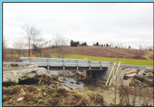
Photo Submitted Traffic is flowing and so is the water on the new Grassy Creek bridge in the Kentontown area of Robertson County. Grassy Creek bridge has been under construction for several months. People in the area are glad all that is left to do now is the cleanup as traffic will pick up as family and friends come home for the holidays
