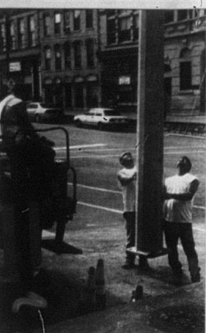
Photo by Charles Mattox. Harley Fleck, left, operates a crane, as Ashley Meyers, center, and Greg Ribickoff, right, identify a new utility pole at the corner of Main and Locust Street in downtown Carlisle.
