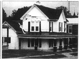
Wind Damage in town
