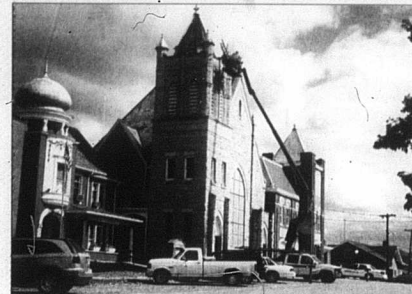
Workers with Adams Roofing and Flashing and Helton Roofing, both of Lexington have been working on the Carlisle United Methodist Church all week.
