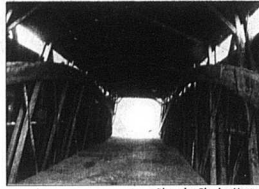
Photo by Charles Mattox This is an inside view of the Robertson County covered bridge at Johnson Creek.
