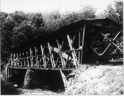
Sideboards have been removed from the Johnson Creek Covered Bridge as renovation continues in an effort to strengthen the deteriorating structure, which was built over 130 years ago.
