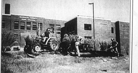
Members of FFA work on the new bus loop at Nicholas County High School.
