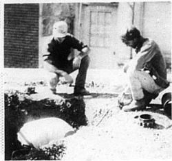
Kinney construction workers and city employees. "Red" Jefferson work on city water lines. Monday, October 28.
