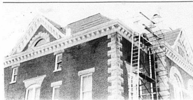
Courthouse roof nearing completion Roofers began installing copper valleys on the courthouse roof Friday, the roof is hoped to be finished by mid to late April.
