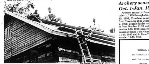
The A. J. Payne Family is refurbishing Loretta and Bill Mann's residence along Highway 32 at Myers Station to look as the structure looked in the days of the Civil War. Payne remodelled the kitchen 19 years ago and did such a fine job, the Mann's asked him to restore their home. The home is full of history. The remains of the Myers family are in a cemetery behind the home on the rail across the railroad track. The home originally faced the track. Mann still has a letter written by a Myers when he was planning for Gold out west. The Myers family is related to G. C. Myers, owner of Carlisle Drug.
