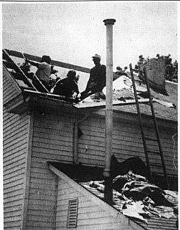
David Hopkins, Ench Doyle and Mike Pryor work to repair the roof of the R. S. and Kay Wilts home on Moorefield Road following Sunday's devastating storm.
