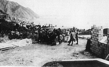
The view of the Caribbean was a bonus as the Kentucky Army National Guard manned a work site to build housing for arms for the Dominica police. The 2014 Engineering Company also took gifts to a nearby orphanage.
