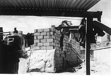
Kentucky Army National Guardsman Jim Cubrath supervised the construction of the arms building being made for the Dominica police force. The guard list includes Major Clint and returned Easter Sunday, April 16.
