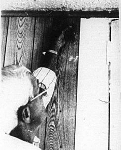
Nicholas County Judge Executive Chuck Smith looks over the newly remodelled room on the third floor of the Nicholas County Courthouse, which has a roof leak damaging the new work. The county's grant application for a new roof, rejected last year, will be revised and resubmitted this year.
