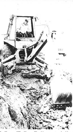
Clay Myner of Clay Myner Plumbing operates a backhoe behind the elementary school Friday to find the collapsed sewer line, which was under a math approximately 12-14 feet of fill dirt. (Photo by Kim Hamilton)
