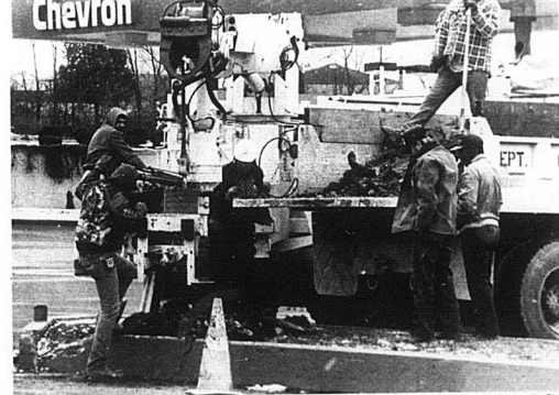
The Carlisle Mercury/Jason Hart Photo The Kentucky Department of Highways drill the hole to set the post for the new traffic lights which will be located in front of Crossroad Chevrolet. According to area residents, the traffic lights will be a relief to parents whose children walk to and from school.
