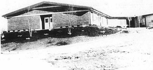
This is the view of the newly constructed Johnson-Mathers Health Care nursing home addition under construction now.
