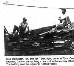
Mike Harrington, left, and Jeff Tyeer, right, owner of Tyeer Construction, Carlsle, are applying a new roof to the Mercury Office. The building is on the register of Historic Places.
