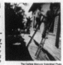
The Carlisle Memory Bank Volunteers work on painting the Bartterville United Methodist Church.
