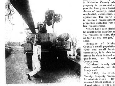
Carlisle Mercury Photo by Rebecca Mullins Layton Gross, an employee of Drifwood Utility Contractors of Paris, spent last Thursday morning replacing 20 utility poles along Upper Jackstown Road. The poles, some of which have been standing from 20 years, have to be replaced after so many years to prevent power outages and accidents caused by poles that are tall down.
