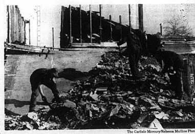
The Carlisle Mercury/Rebecca Mullins Photo High school students (from left) Sam Jones (center) and David McLean worked Saturday to dispose of rubble at 382 Main Street. The house was torn down recently by an ice storm, according to Carlisle City Police Officer Jerry Bloomfield.
