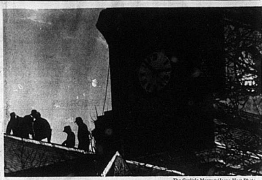
The Carlisle Mercury/Dean Hart Photo Workers toiled to repair the roof of the Nicholas County Courthouse last week. According to Ernest Sosby of the Nicholas County Historical Society, the courthouse is over 100 years old this year.
