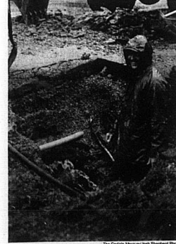
The Carlisle Mercury Staff Staff Photo City worker and city fire chief Tommy Crawford uncovers a water line leak Wednesday afternoon that left several homes without water for most of the morning. The centrifugal break in the water line, a result of settling and ground movement, was quickly fixed by the application of pipe clamp.
