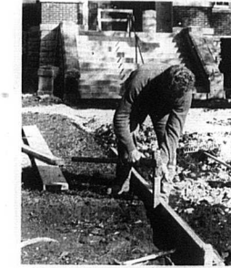
Employees of the County Concrete Company busy set the borders down for the foundation to a new sidewalk to the courthouse. In keeping with several people's request, the sidewalk has been extended to the Veterans Memorial monument in front of the courthouse. The court and the company reached an agreement to have the work done in lieu of lease payment.
