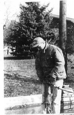
The Carlsle Mercury Staffed Photo City worker and Carlsle Fire Chief Tommy Crawford jackhammers open a section of Douglas County to get at water leak in the area. A leak from one of the pipes was caused by possibly a stress break in the line or by simple wear and tear on pipes upwards of nearly 40 years old.
