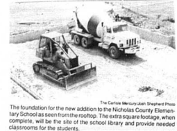
The foundation for the new addition to the Nicholas County Elementary School as seen from the rooftop. The extra square footage, when complete, will be the site of the school library and provide needed classrooms for the students.
