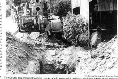
Bath County Water District workers use a crane to drill a unit into a ditch line in front of the entrance to Cassidy Creek Road in Myers Station.
