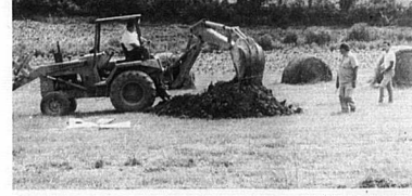
The Carlisle Mercury/Job Shepherd Nicholas County Fill Supervisor Phillip Howard collects soil samples for Steve Burns of Endicott and Associates and George Attanasio of who will be performing lab tests on the soil. This work is in preparation of the state Landfill Closure plan.
