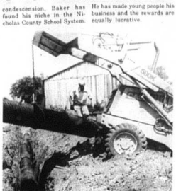
Gayle Vandendorp oversees placement of storm sewer pipes running along the railroad tracks near the entrance to East Union Road in Carlisle.
