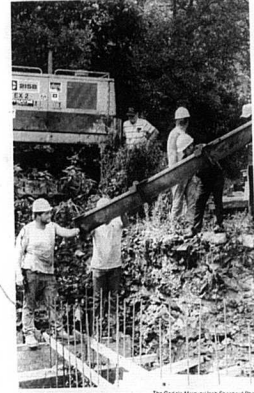
Judy Construction workers out of Cynthiana begin pouring the concrete base for a new bridge on Stoney Creek Road. The new bridge is planned to span three feet above road level to prevent wash outs during Creek flooding.
