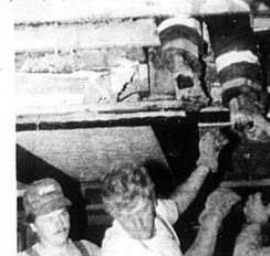
The Carlisle Mercury/Pam Boukris Photo The Nicholas County Fire Department responded to an early Wednesday morning fire at the residence of Robert and Paula Satter of 2200 Spring Court in the city. The fire, which started in the attic portion of the house, Nicholas County Fireman Sam Reynolds gives Fire Chief Mark Hughes a boost up the attic as Robert Hughes looks on.
