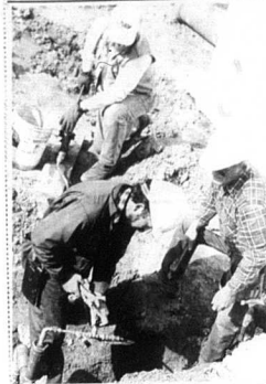
The London Bridge Construction Company have been taking more pressure tests than anticipated when problems with the piping to the new sewer plant began to occur. Plant supervisor Gene Kelley assisted construction workers by adding water pressure on one of the pipes, testing its ability to hold pressure. The project is entering its fifth week of delay.
