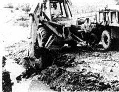
The Carlisle Mercury Josh Shepherd Photo City workers open and widen a water drainage ditch next to the sewage treatment plant to accommodate the rise in water flow from the nearby trailer park.
