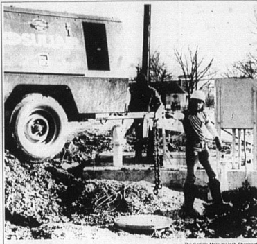
Nearly finished Workers install water pumps that will pump sewage through the city sewer plant. The plant is expected to be operational by next week.
