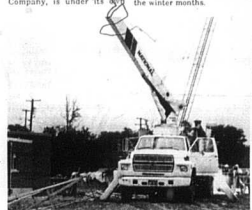
The Carlisle Mercury/Josh Shephard Photo Sewer plant construction for the City of Carlisle is halfway complete, Gene Kelley, construction supervisor and liaison to Carlisle City Council, said. Estimates from workers say the construction could be complete long before the March 1 deadline.
