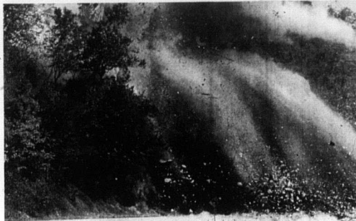
Several controlled explosions rip out the side of the campground hill in Myers as part of the new bridge work on Flemingsburg Road. Tom Hite of the Rose Construction Company, the primary contractor for the work in Myers, said work should be completed by the end of 1990.
