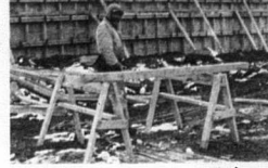
Workers continue to make progress on the new branch bank of the Deposit Bank of Carlisle.
