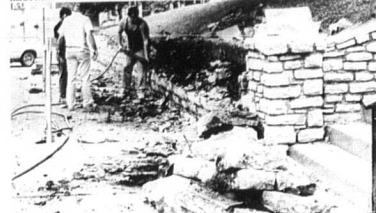
Workers for Donald Robinson Masonry take apart the Nicholas County Courthouse creek stone wall facing Main Street to straighten the wall foundation. Workers are saving most of the creek stone to be used to piece the wall together again after work on the foundation is finished. Josh Shepherd Photo
