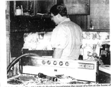
Nicholas County Fire Chief Mark Hughes investigates the cause of a fire at the home of Harrison and Mary George on Moorefield Road Monday morning. Hughes said the fire was possibly caused by a combination of old electric wiring and high humidity. Volunteer fire fighters spent time removing burnt insulation and venting out smoke from the house attic. Josh Shepherd Photo
