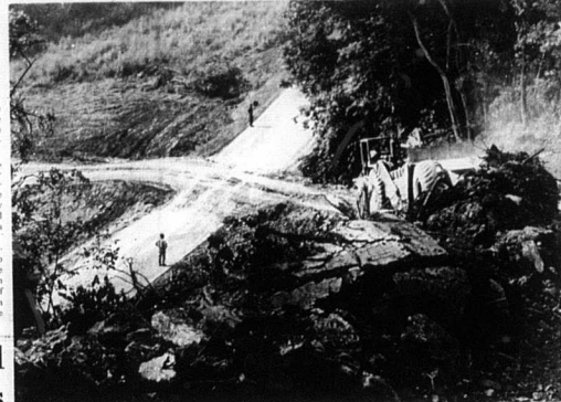
Construction has begun on a new bridge to replace the Licking River bridge on Myers Station Road (KY 32). Plans call for the hill above to be leveled and the bottom near the Licking River to be raised. The Federal project has been planned for three years and is slated to be completed by the spring of 1990. — See additional photo on page 15. — Josh Shepherd Photo.
