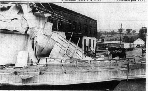
The sky is falling, but a strong wind did take the roof on Heid and Vice for a ride on the evening of July 10, and eventually set the top end for a rest in the street. Workers were busily working to remove the debris the next morning. Power was restored to the area and Heid and Vice was open for business. - Heather Mathes Photo.
