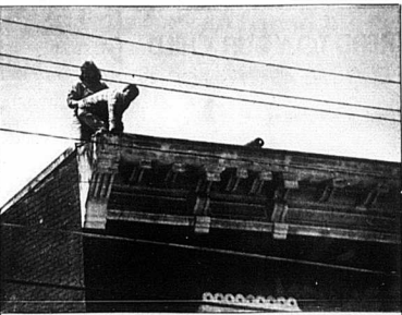
Dorn and Wayne Manley are shown working to repair the roof of the old Nicholas County Jail in Carlisle. The Carlisle - Nicholas County Senior Citizens Center is scheduled to be relocated to that building about July 1, if all goes according to plan. — Marsha Livingston Photos.
