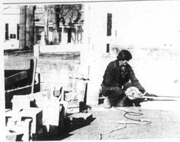
Kenny Thersberg builds up the concrete wall parallel to Kelly's IGA for Mr. Gayle Kelly — photo by...
