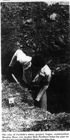
The city of Carlisle's water project began construction Monday. Here, city worker Dale Faulkner helps lay pipe on the first line beside Old Paris Road. (City/Steve Pugh)
