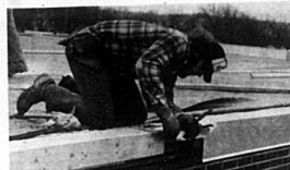
Philip Bueck of 848 Builders puts the finishing touches on the roof of Nicholas County Elementary School...
