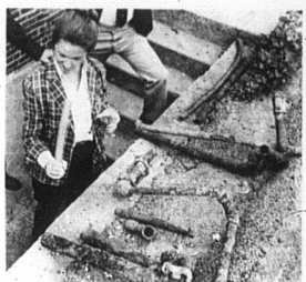
Diane Roberts of the HUD Office in Louisville examines the new kind of gas pipe proposed for the Carlisle gas pipe replacement project. HUD is one of the funding agencies. Also shown are examples of the old gas pipe, corroded and out of use. — Mercury photo.
