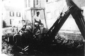
Community Park construction The Carlisle Community Woman's Club is constructing a community park behind the old L&N depot building. Construction began recently and Johnny Hamilton is shown here with the backhoe. Completion is planned for early fall and it will be open to the public. — Photo submitted.
