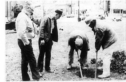
A spectator sport The smartest part of this job was finding the sewer line. The line stopped up in the courthouse a few days ago and Courtney Gunn (second from left) walked out on the front lawn and said "dig here." Three feet down, Carl Crawford (second from right) and Gary Corder (far right) came out right on top of the line. On the left is Bill Sams, who described himself as an "observer." The men digging are employees of Clay Mysner Plumbing and Heating. — Mercury photo.
