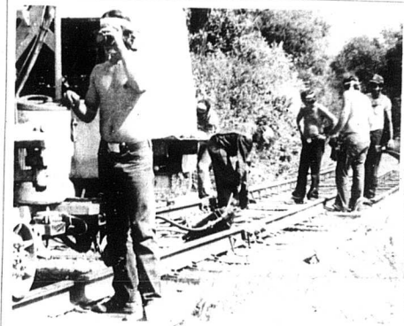
...All the live-long day A cool drink of water provided a pleasant pause for this TTI employee as he and fellow workers continued repairs on the railroad tracks near Carlisle Monday afternoon. — Mercury photo.
