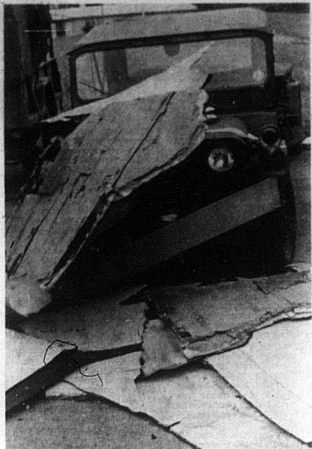
Armory damaged A section of what was once the roof of the National Guard Armory wound up across this jeep after Sunday's violent thunderstorms tore through the county. — Mercury photo.
